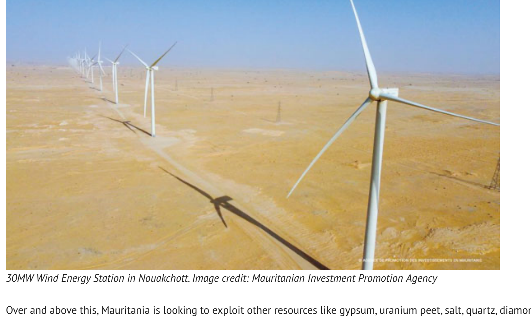
30MW Wind Energy Station in Nouakchott. Image credit: Mauritanian Investment Promotion Agency
